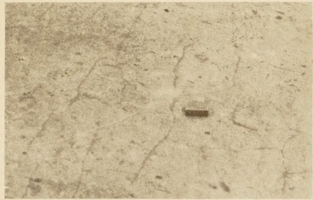
FIGURE 1.—CHARACTERISTIC SHRINKAGE CRACKS DEVELOPING IN THE MARL BASE AS IT DRIES OUT AND HARDENS
